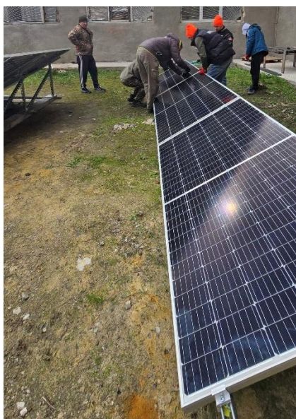
Figure 3. Assembled Solar Field
